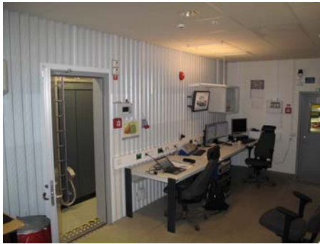
(c) Control room
