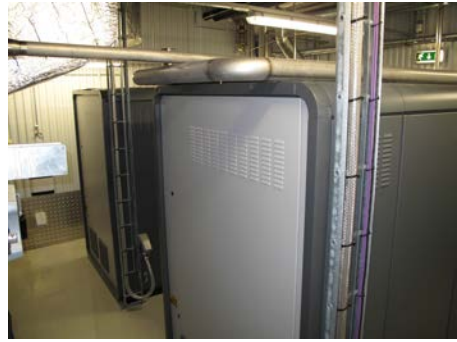
(b) Screw compressor room.
