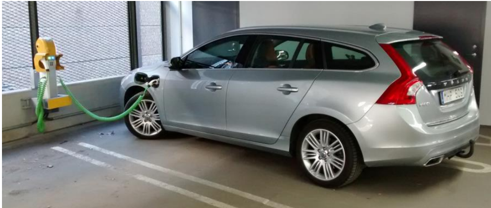
Figure 4: Volvo V60 PHEV charging with a Garo charger at the Linköping University Hospital parking garage.
