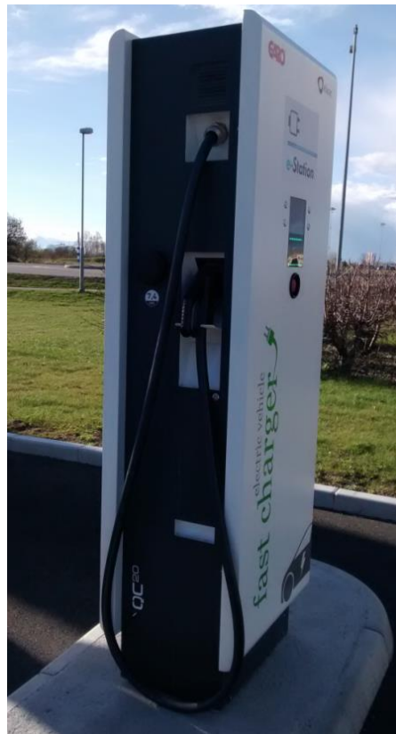
Figure 2: The Garo QC20 fast charging station, outside Engströms Bil, Linköping.
